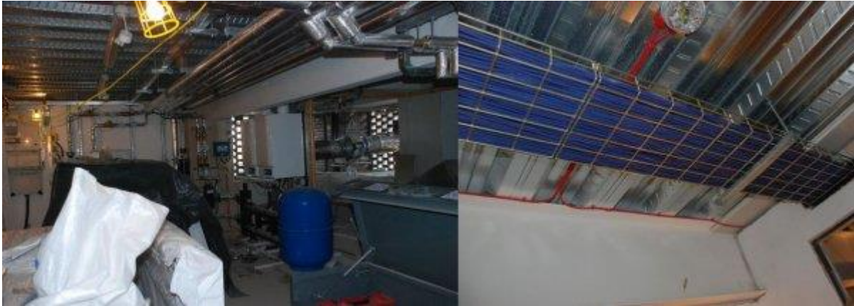
Left - the boiler room; right - IT cables
